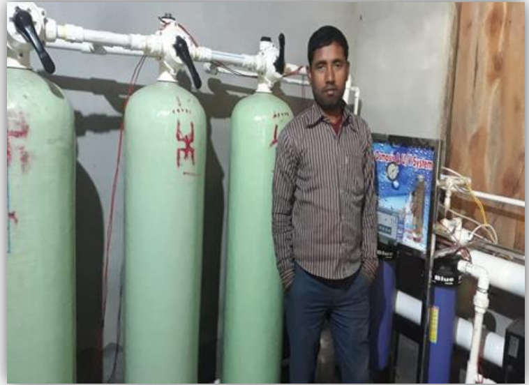
Bikash at his Water Purification Plant
